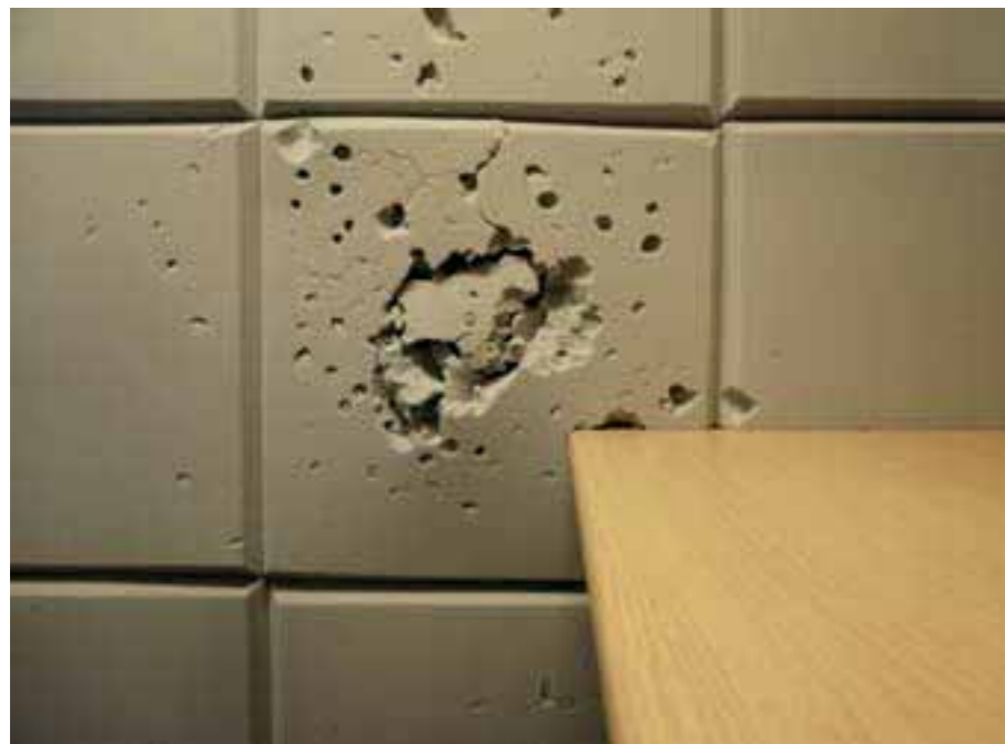
Torn soundproofing in a Cobham AVL studio
